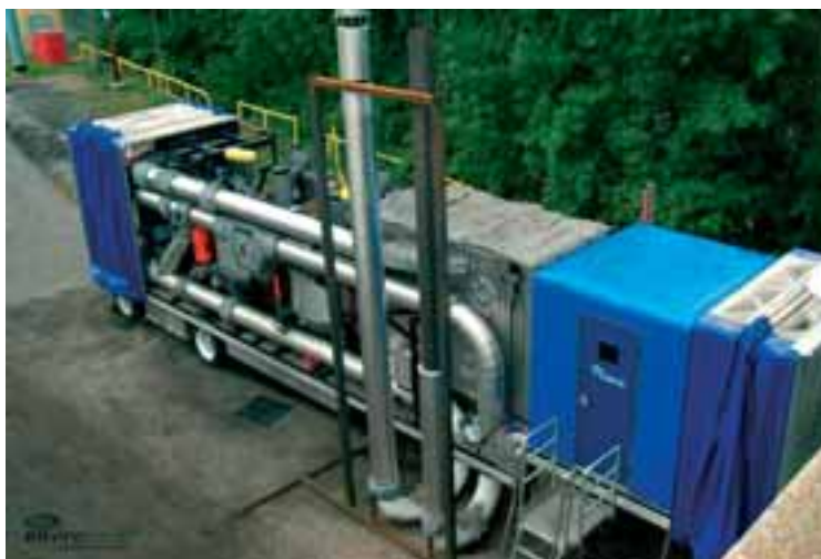
The EnviroScrub Technologies Mobile Unit running at the Potlatch Paper Corporation facility.
